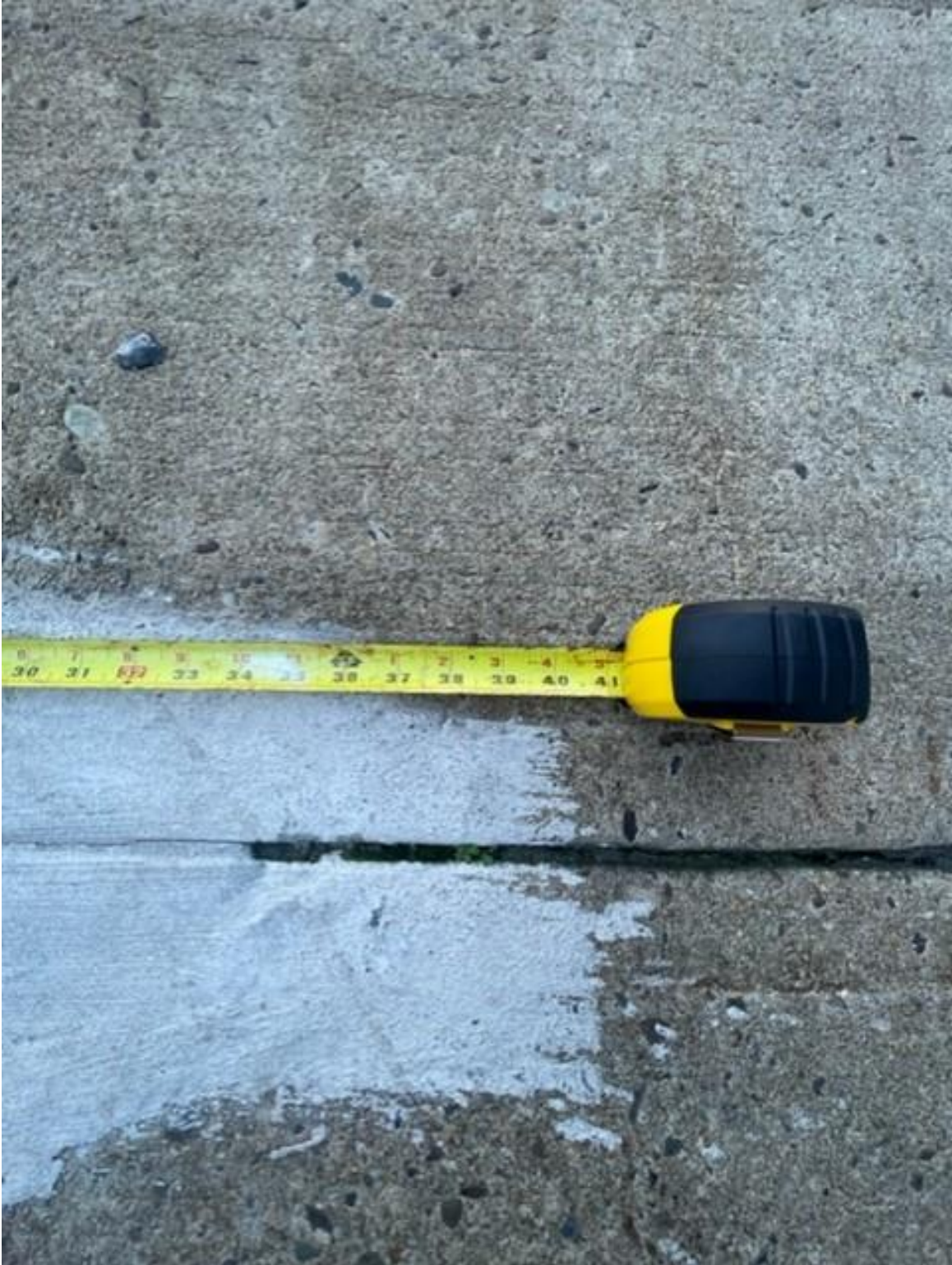
Repair measured 40" in length.
