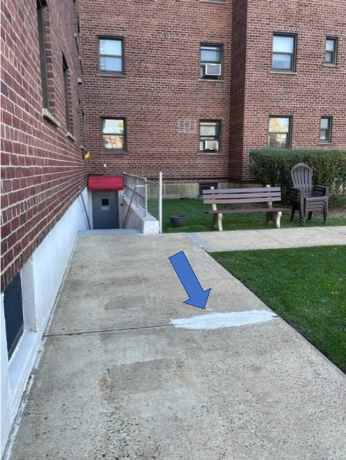
Damage to walkway in the rear of building 3, which allegedly caused claimant to fall. This photo depicts the walkway after repair was done.
