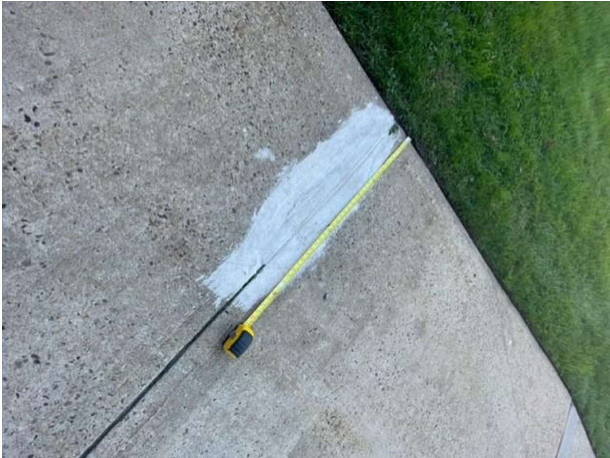
Repair measured 40” in length.
