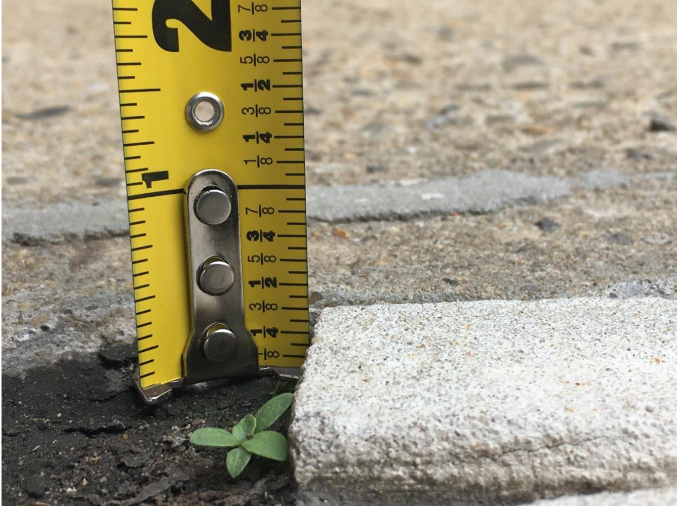
Photo taken by Peter himself just after the incident, before the walkway was repaired
