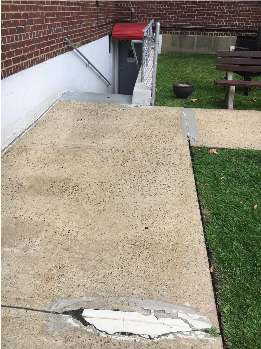
Photo taken by Peter himself just after the incident, before the walkway was repaired
