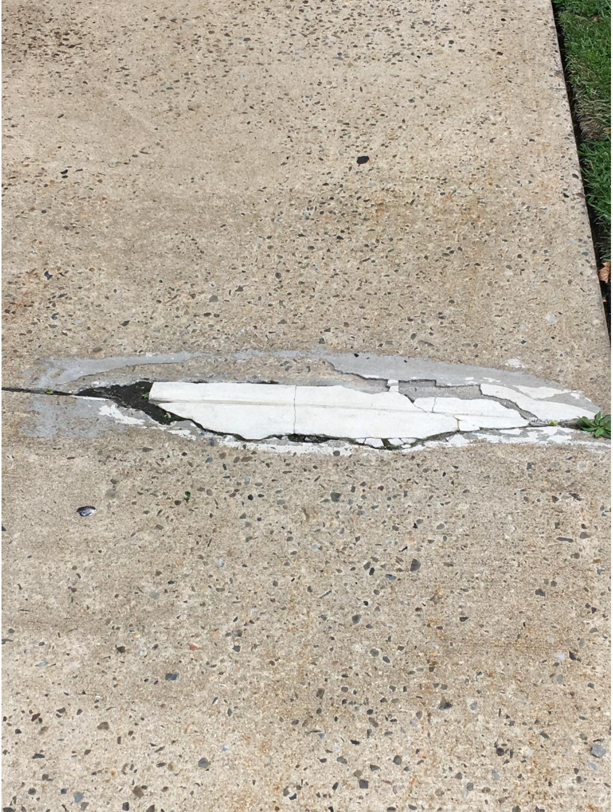
Photo taken by Peter himself just after the incident, before the walkway was repaired
