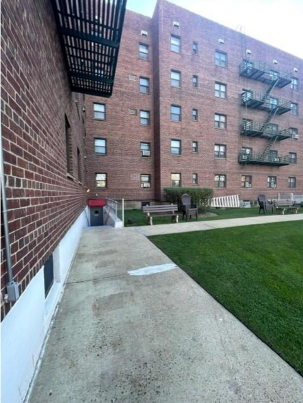
Damage to walkway in the rear of building 3, which allegedly caused claimant to fall. This photo depicts the walkway after repair was done.
